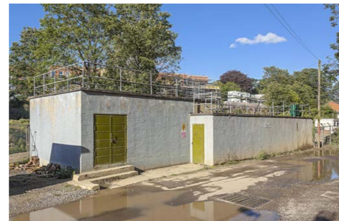
Severn Trent sewage pumping station – under review.
