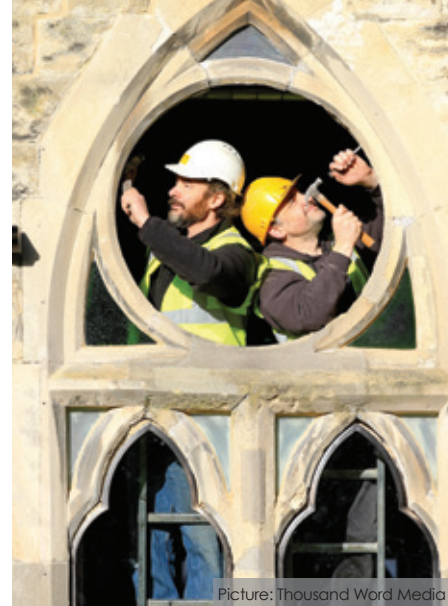
Dave Lush and Tim Clevely from DLS Church Windows at work in Lansdown Hall
