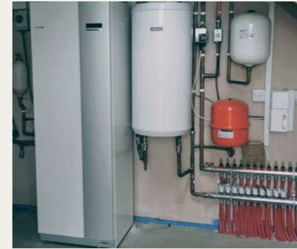
Ground source heat pump
